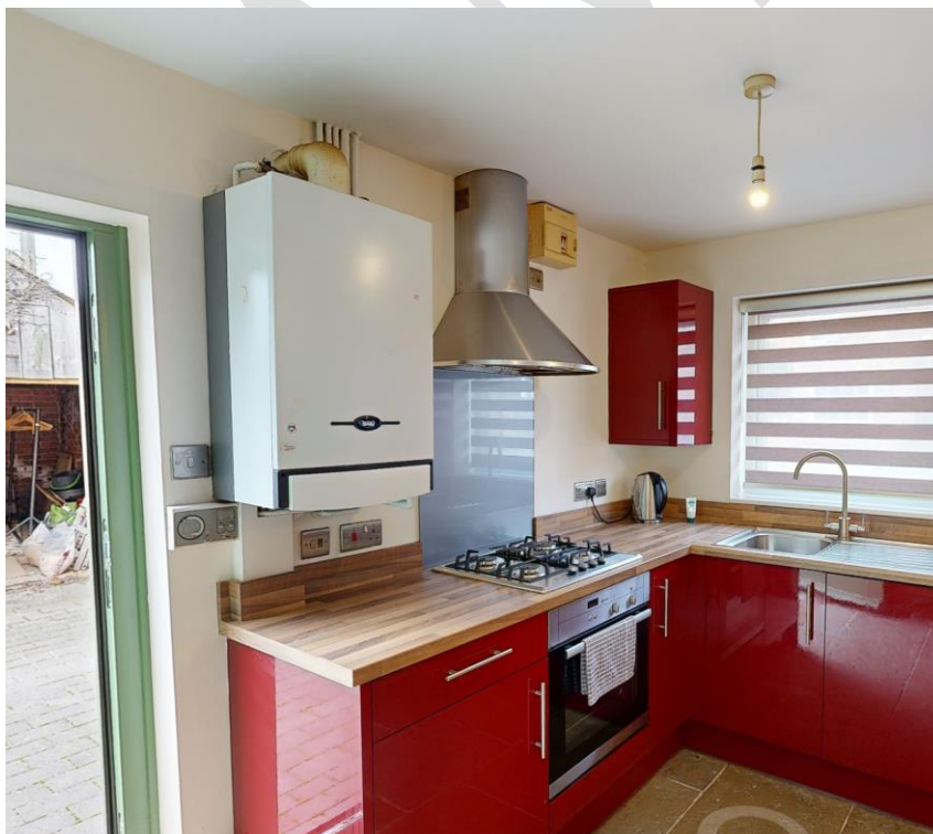
Figure 1: Current gas boiler in kitchen
