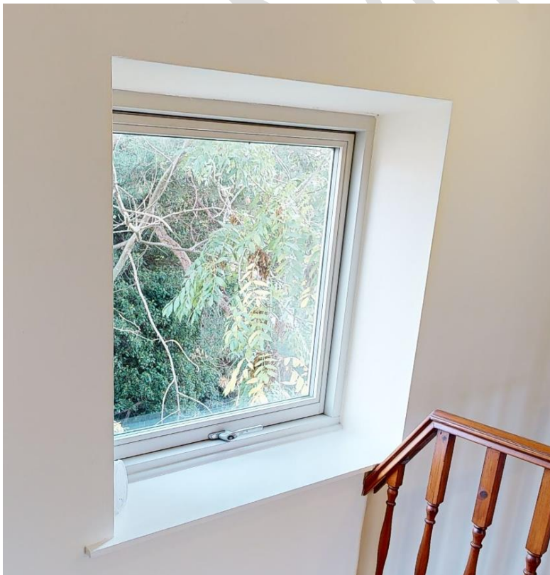
Figure 3: Image showing good quality double glazed windows, installed in 2015 with original documentation supplied. Note lack of trickle vents and depth of dry lining.
